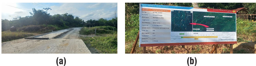
Figure 31. (a) Repairing the road connecting Riko-Bukit Subur, (b) Repairing plan of the road connecting Riko-Maridan (Photo credit: Maulidia Savira Chairani and Moh. Syahrul Irfan Fahmi, 2023)
